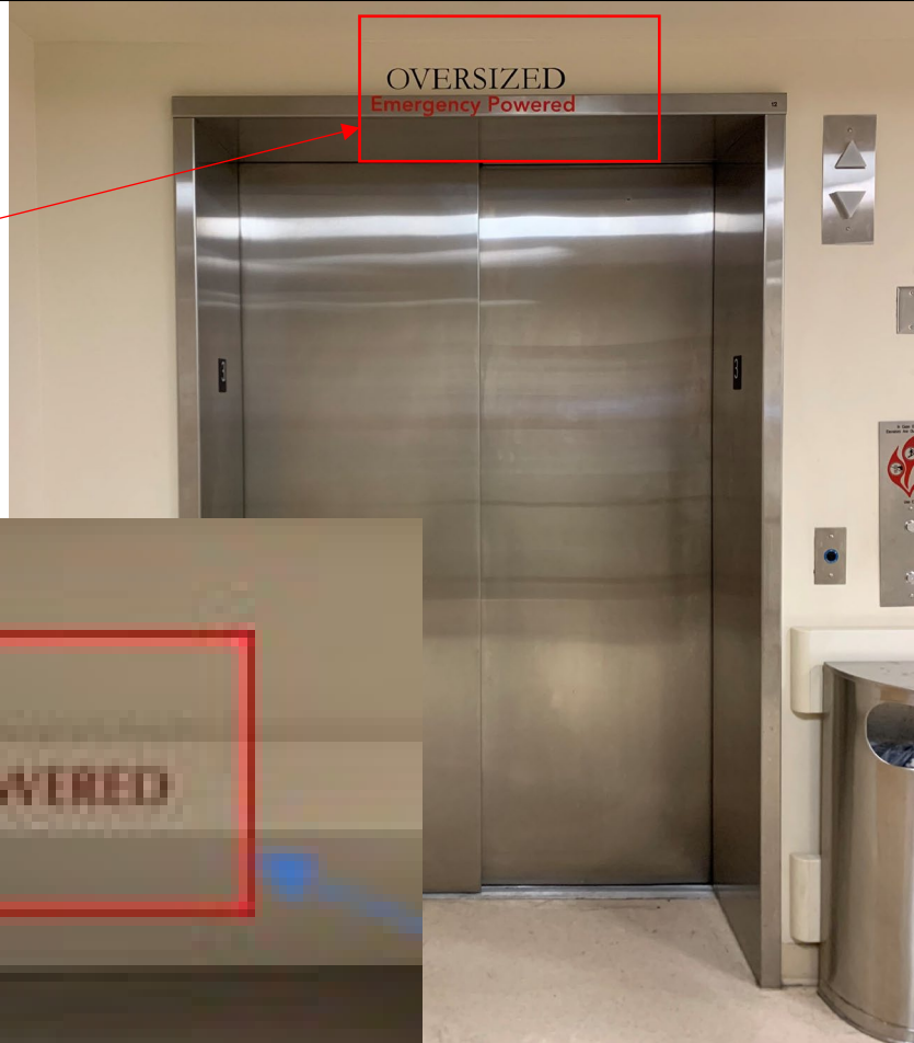
Elevator 12 South Tower (Oversized Elevator)
